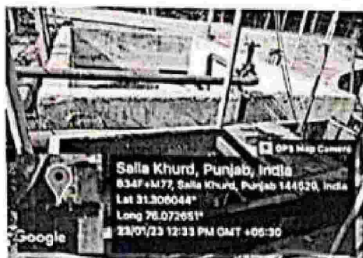
Final Outlet of ETP
